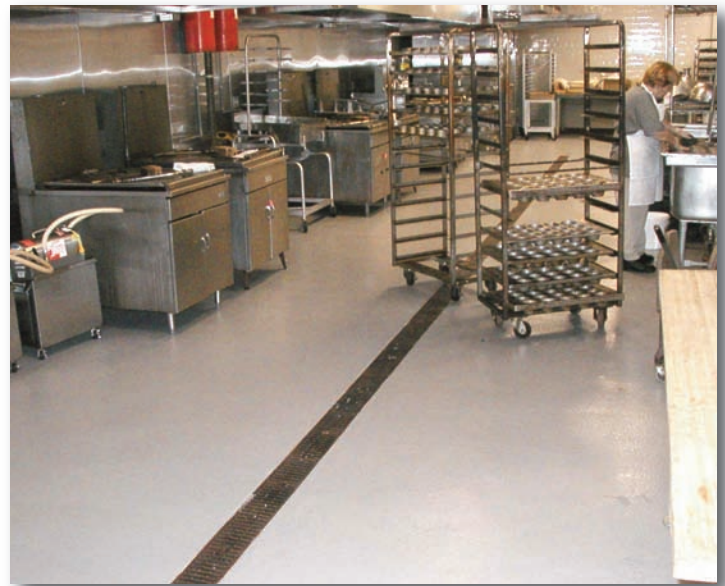
Stonhard replaced Hyatt's problematic tile floors with Stonclad UT, resulting in a seamless, easy to maintain floor.
